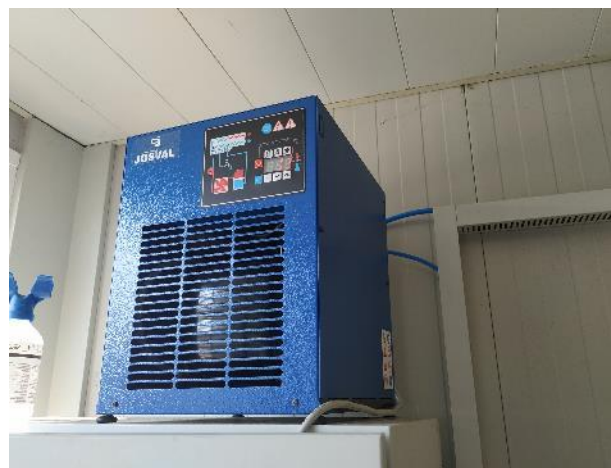
Dryer for the pressure line
